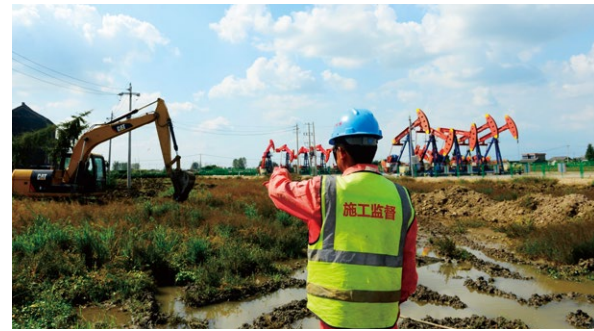
④ Excavation operation for land reclamation on the Cangxi 3-9 platform of the East China Petroleum Bureau Taizhou Oil Production Plant
