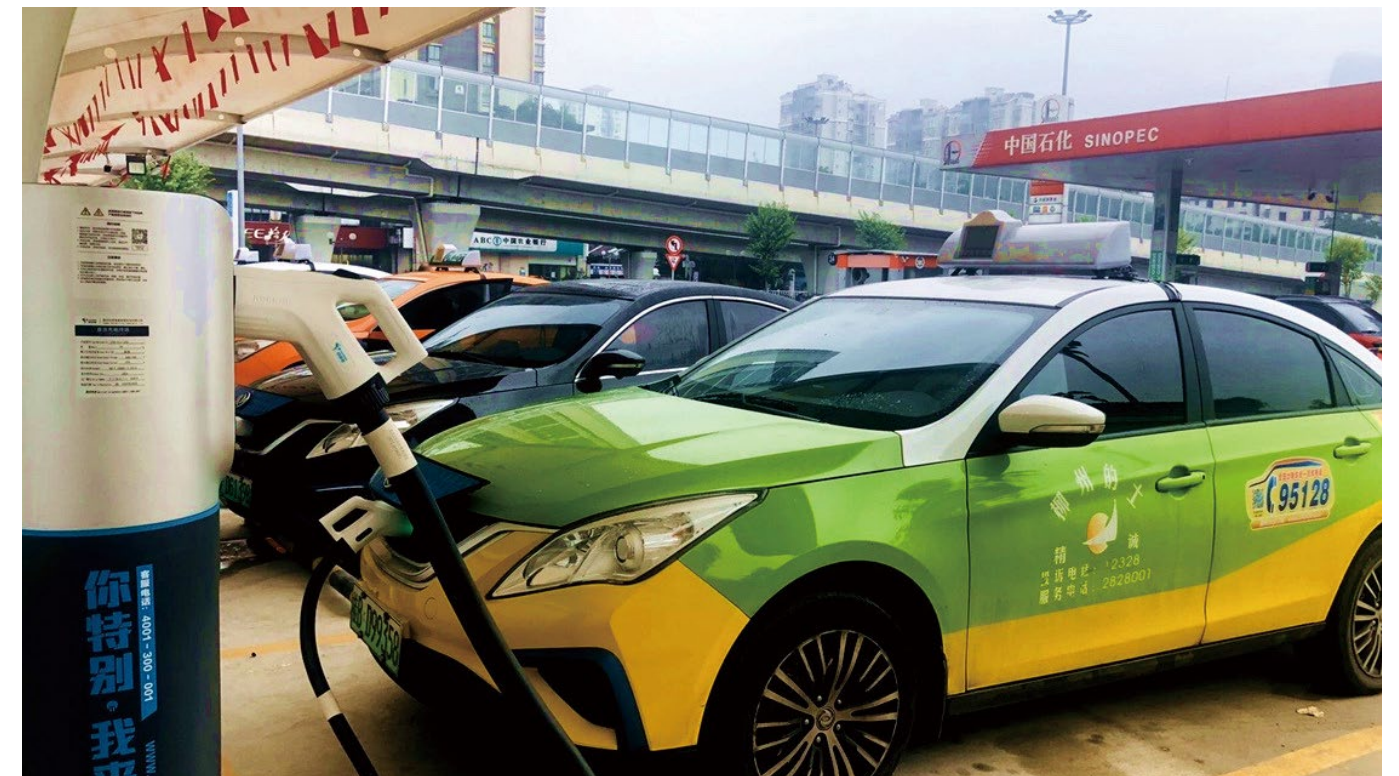
Providing fast charging service to new energy taxis at Sinopec charging stations
